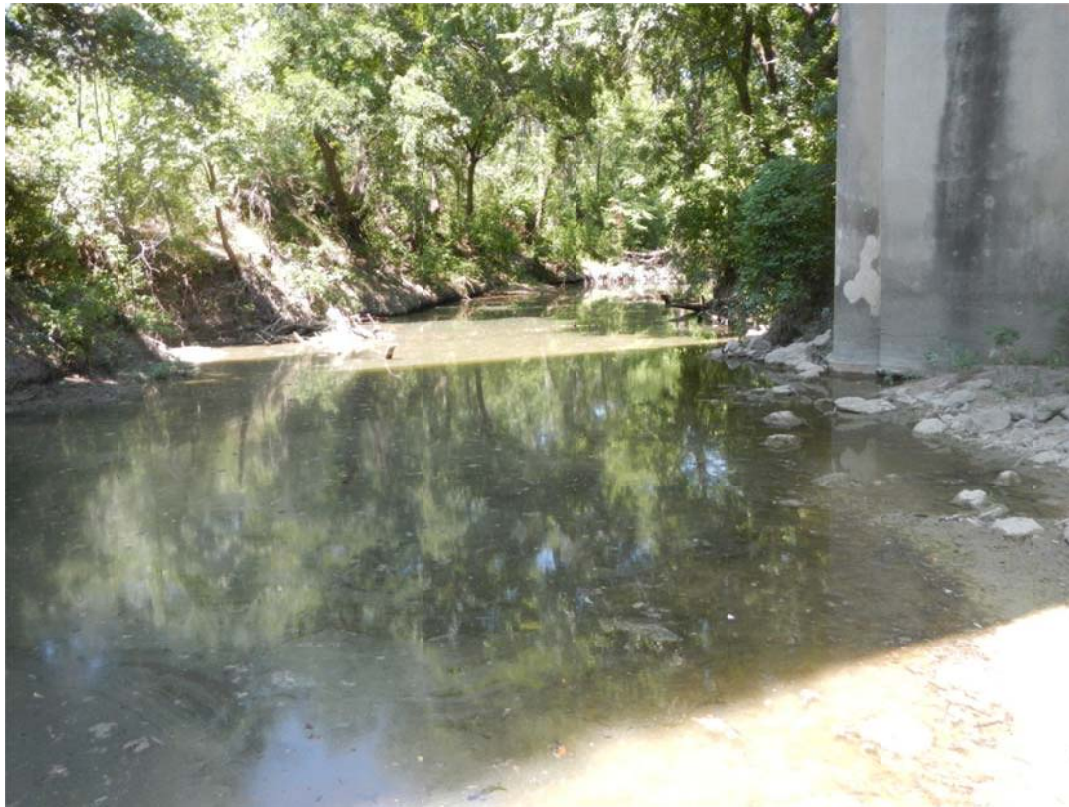
Figure 2-6: SH 71 Bent in Onion Creek due to Eroded Banks
