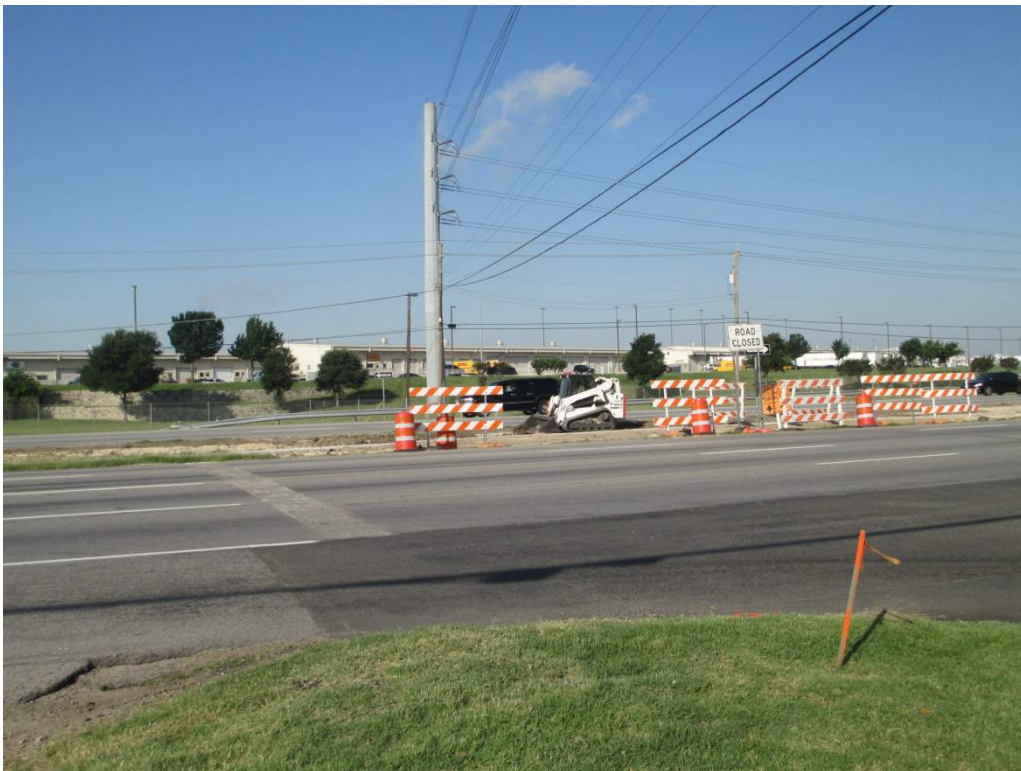
Setting view, south side of SH 71 from Shapard Lane, camera facing south
