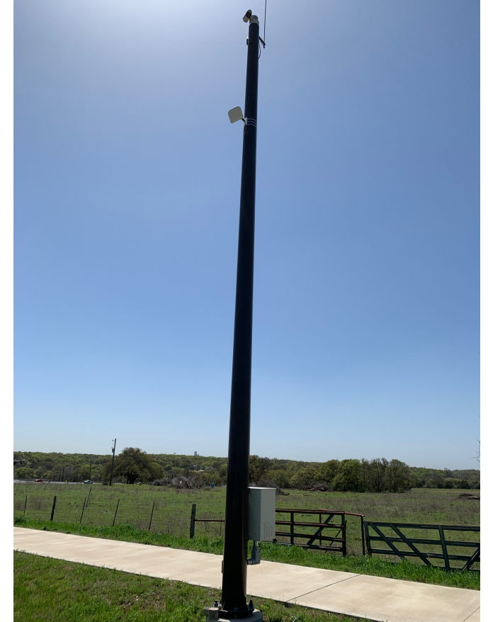
Closed Circuit Television (CCTV) and Radar Vehicle Sensing Device (RVSD)
