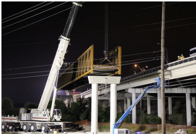
First span of 525-foot bike/ pedestrian bridge now in place over Union Pacific tracks southbound (April 9)
