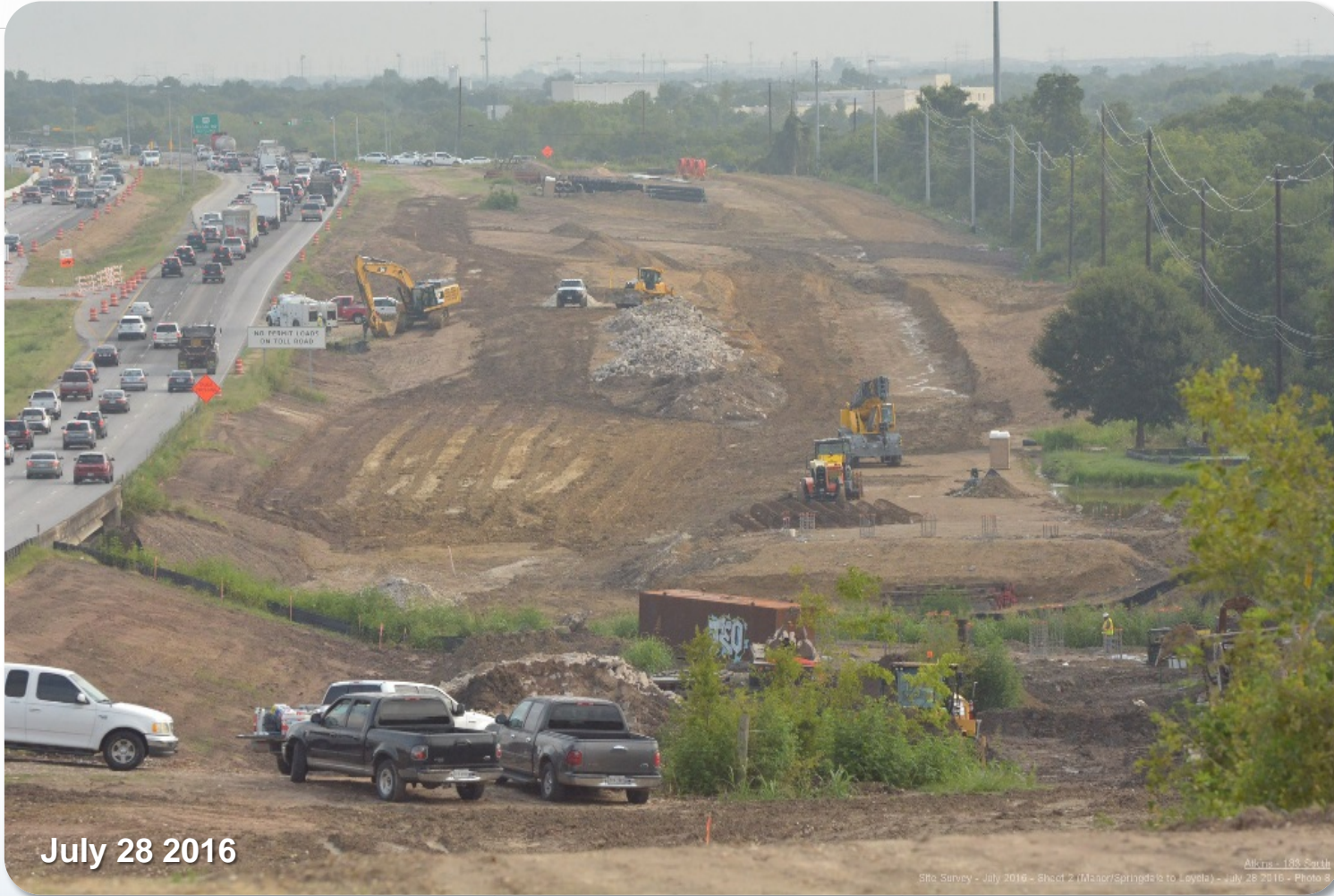
Construction Worksite – Northbound General Purpose Lane at Northbound Main Lanes – Walnut Creek (Facing North)
