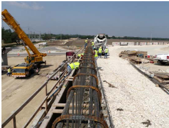
Placing concrete at a back wall for the 183A bridge over Hero Way
