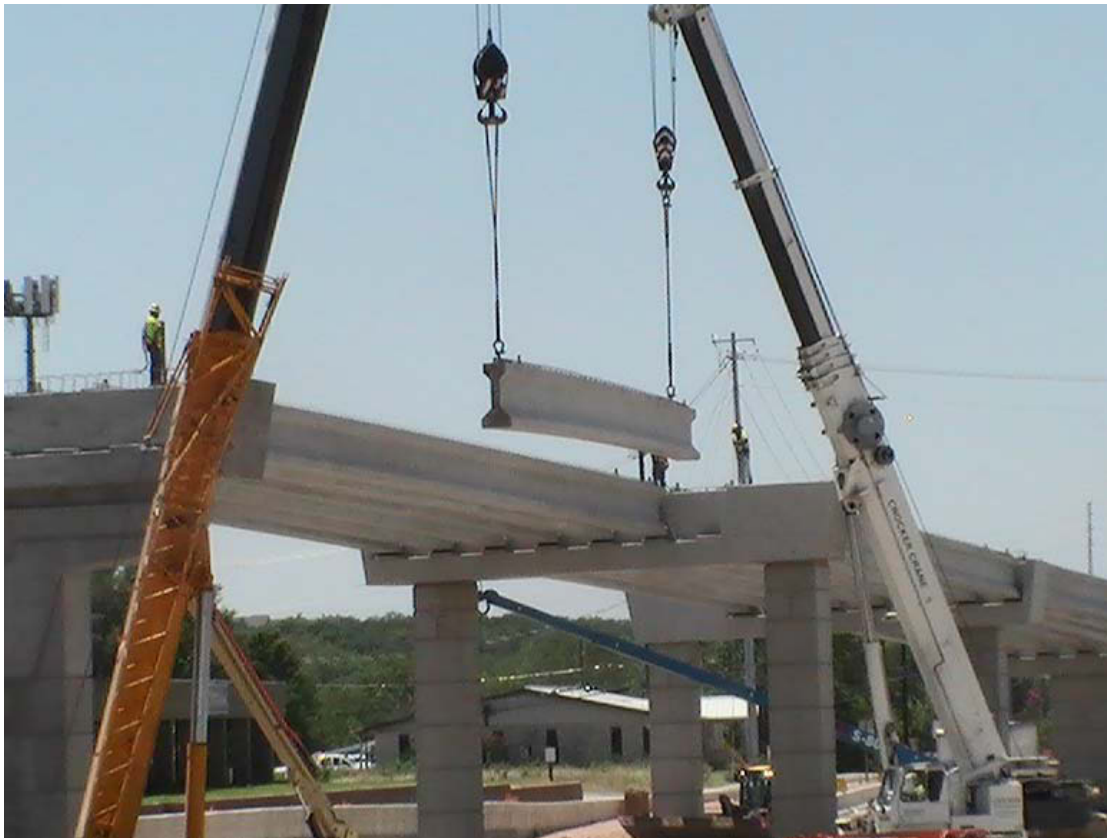
Setting of beams at the south to east direct connector [taken June 14, 2011]
