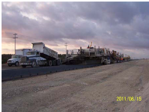
Placing concrete for paving on the mainlanes north of Crystal Falls Parkway
