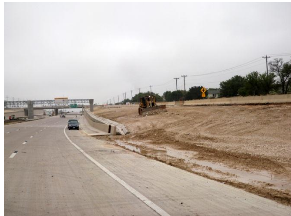
Grading the slope in the northwest corner of the Scottsdale Drive bridges
