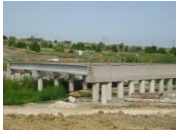
Construction of the westbound frontage road bridge at Tributary #1C (Looking Northwest)
