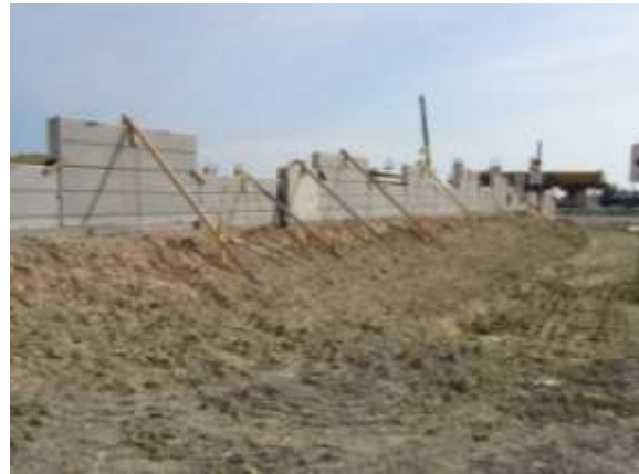
Erection of Wall S3-01 for the eastbound mainline west of SH 130 (Looking West)
