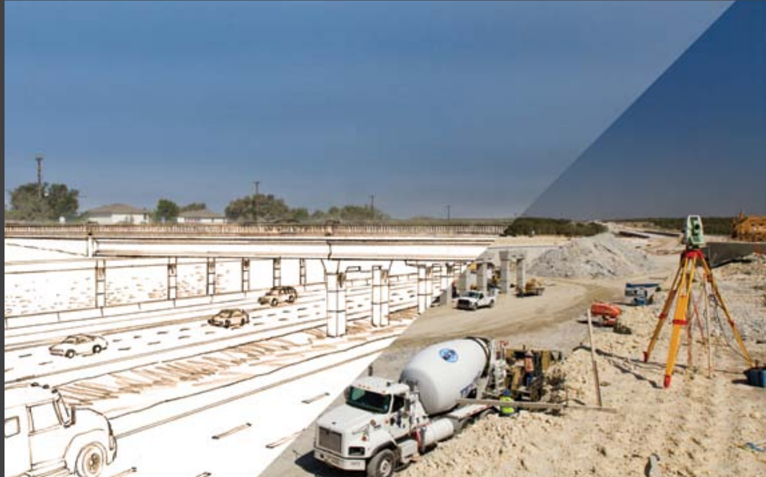
CONCEPTUAL 183A AND ACTUAL WORK ON SCOTTSDALE DRIVE INTERSECTION 183A NORTHERN EXTENSION PROJECT - OPEN 2012
