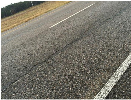
Observed Longitudinal Cracking
