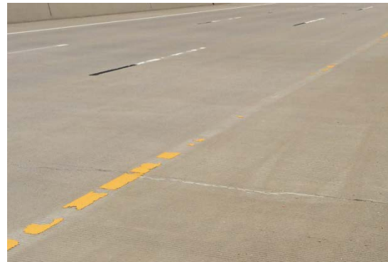
Observed Pavement Marking Fading
