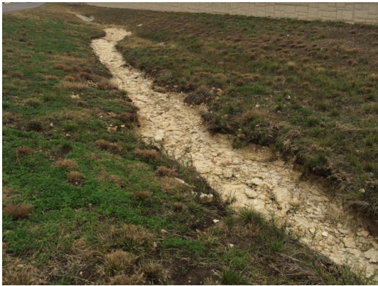
Erosion between SBML and SBFR
