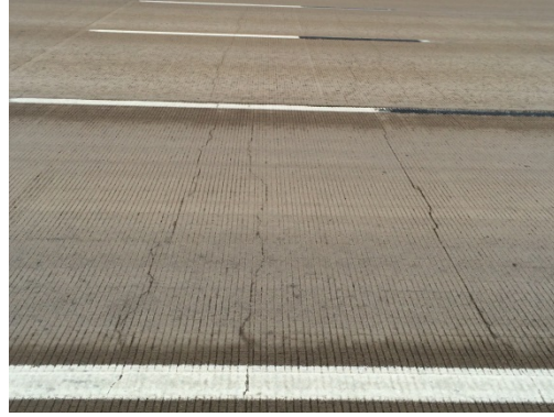
Observed Transverse Cracking
