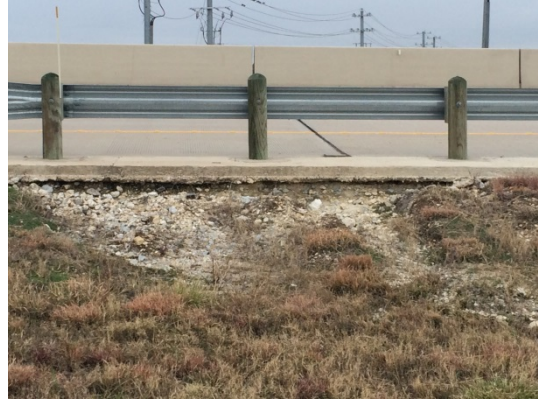
Erosion behind MBGR on SBML
