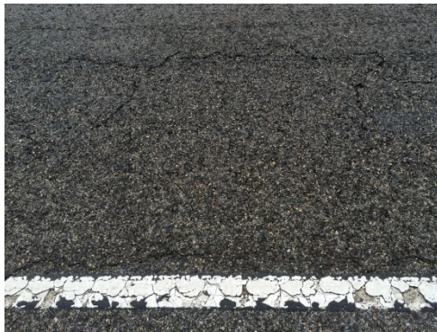
Observed Pavement Marking Cracking
