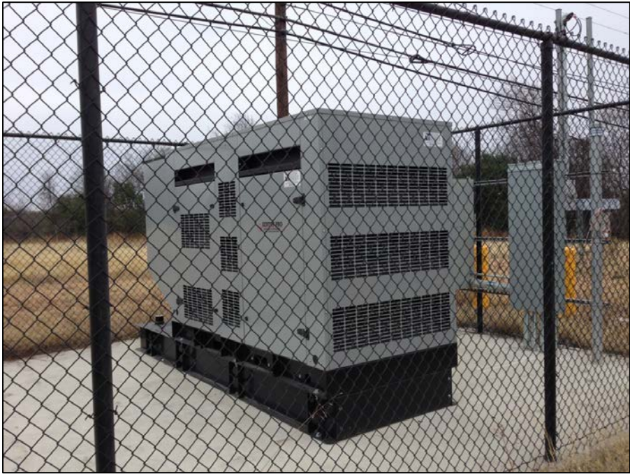
Emergency generator that serves both WNDC and SEDC Ramp toll locations
