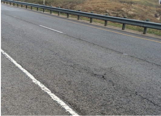
Observed Longitudinal Cracking
