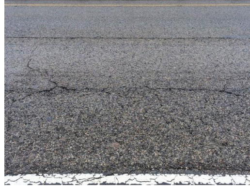
Observed Fatigue Cracking
