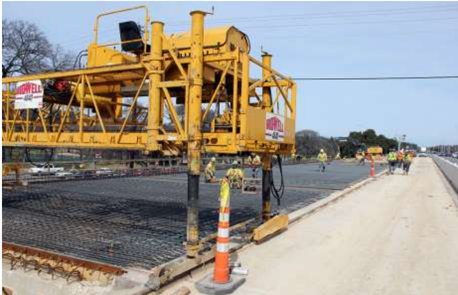
Installing Bridge Deck Rebar on Southbound Enfield Bridge for Concrete Deck Pour
