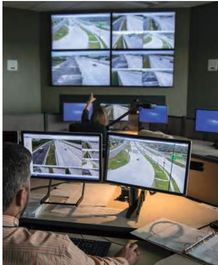
This operations center will be the control center for the MoPac project
