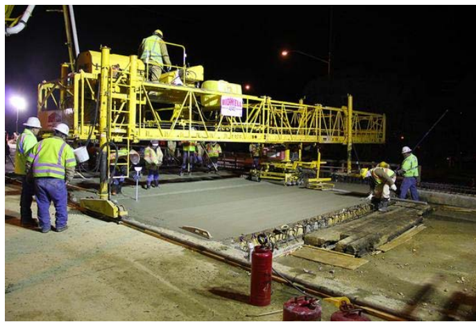
Workers pour the concrete deck for the expanded southbound bridge at Enfield (February 5, 2015).
