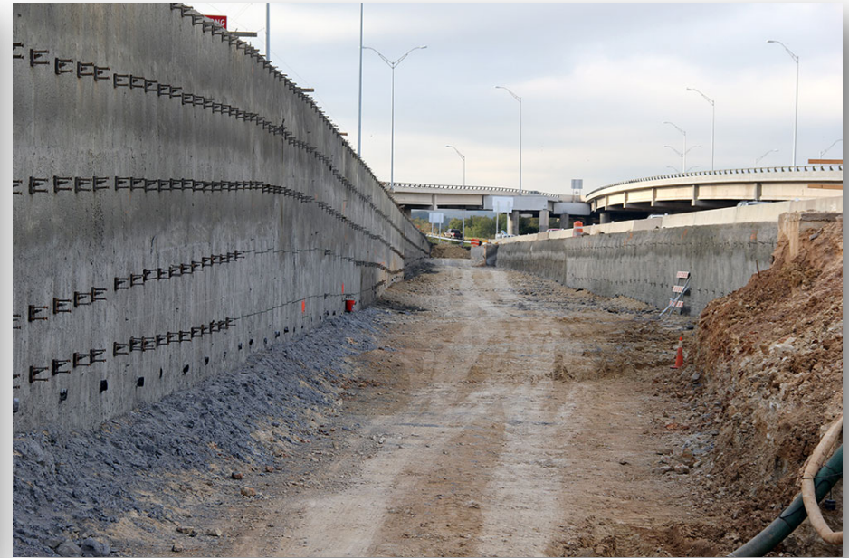
Excavation and Retaining Wall Construction for Cesar Chavez/6 th Street NB Entrance Ramp
