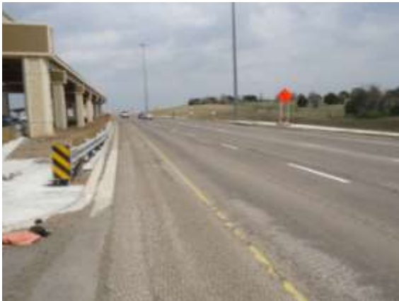
CTMC has milled the eastbound frontage road for the final asphalt course at SH 130 (Looking East)
