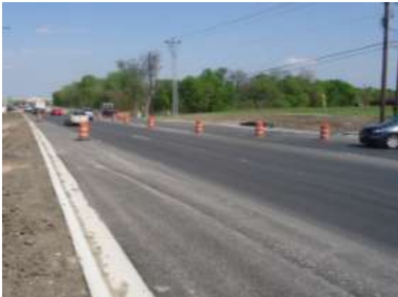
Crews work on transitioning the project back to existing US 290 (Looking East)
