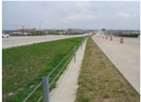
CTMC continues installation of the median cable-barrier (Looking East near Springdale Road)
