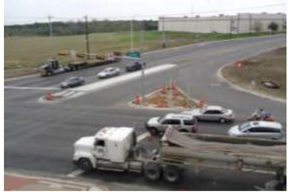
Many concrete islands remain to be completed (Looking Southeast at Giles Road)
