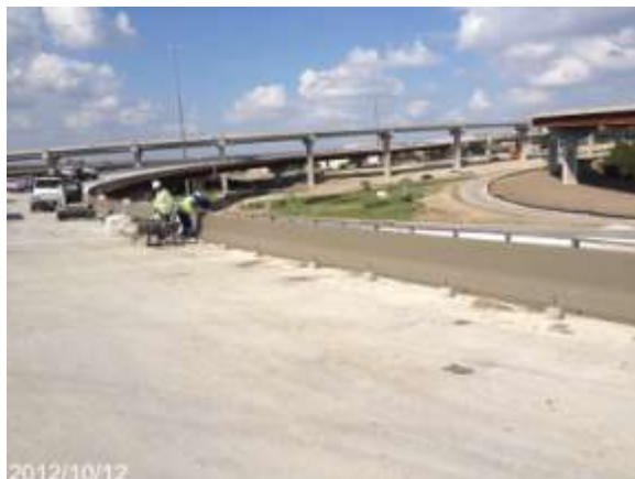
Placement of T501 Rail on west to south Direct Connector (Looking North)
