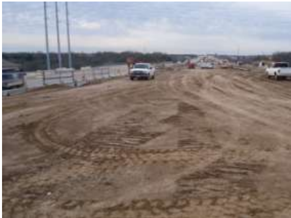
Earthwork embankment for the eastbound mainlane west of Arterial A (Looking West)
