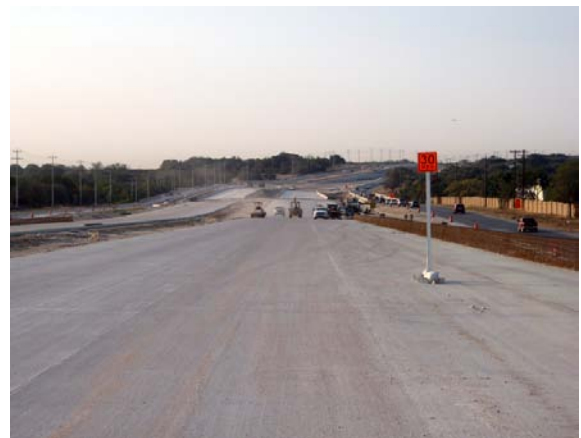
Main lane concrete pavement from Crystal Falls Parkway to Block House Creek
