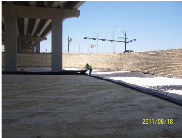
Preparing for rock lining of the stormwater detention pond south of Crystal Falls
