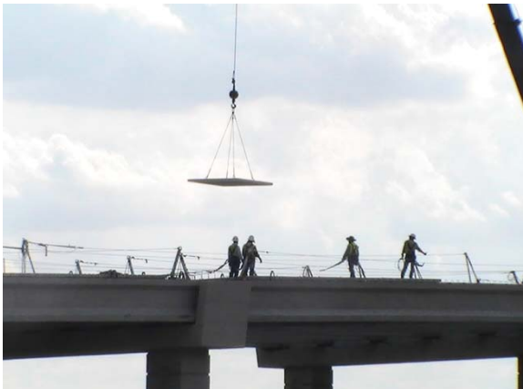
Setting deck panels on the South to East Direct Connector (Looking South)
