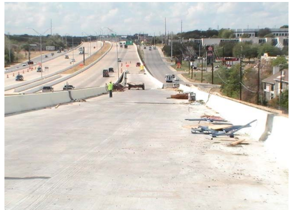
Roadway surface work on the West to North Direct Connector (Looking North)
