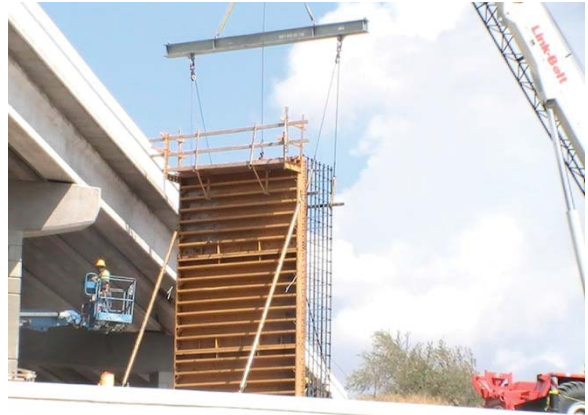
Column steel and formwork on the South to East Direct Connector (Looking North)
