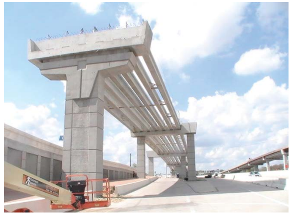
Southbound US 183 on ramp under the South to East Direct Connector (Looking North)
