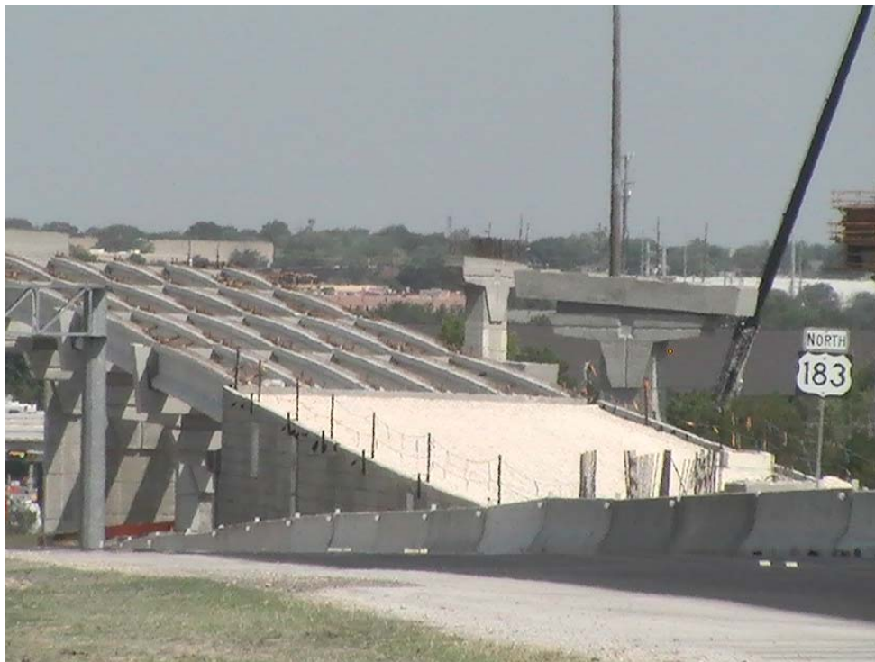
West to North direct connector looking north (Taken 7/6/2011)
